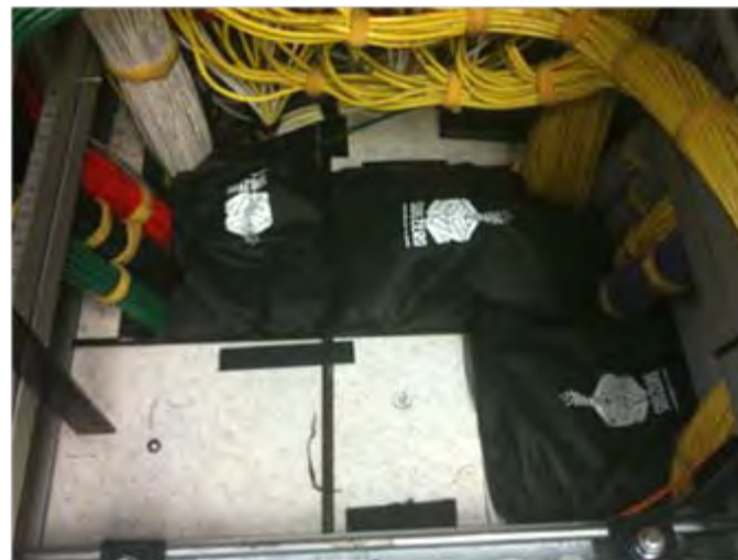
Sealed cable penetration
