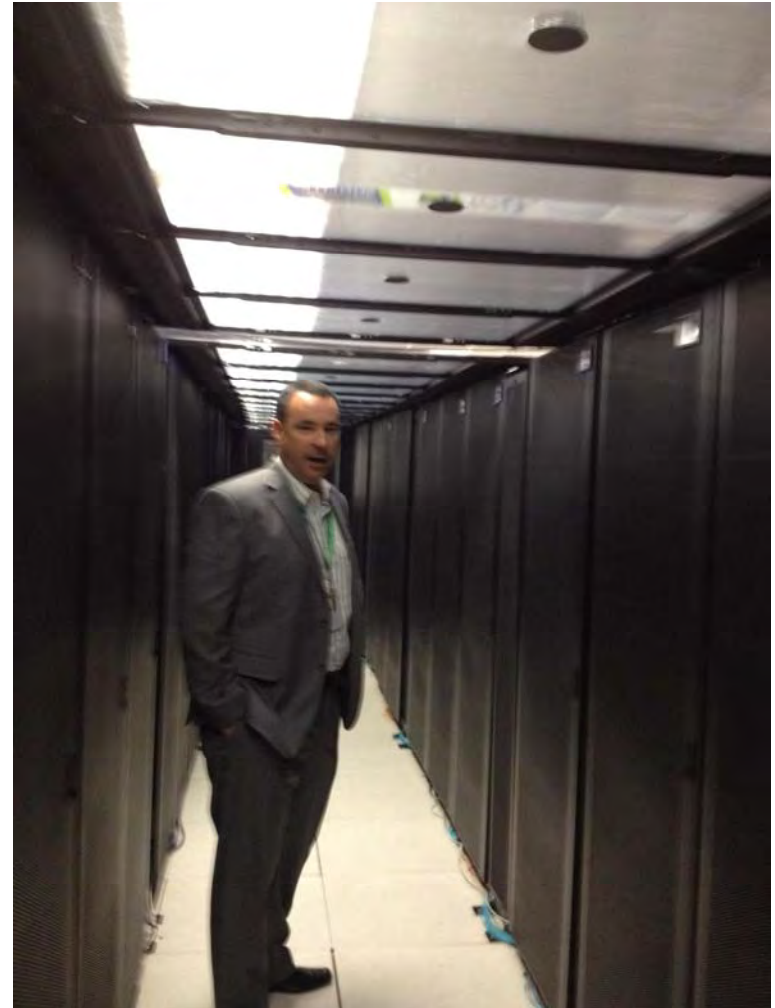
APC Hot Aisle Containment (with in-row cooling)
