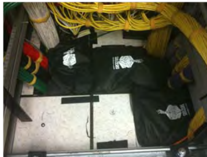
Sealed cable penetration
