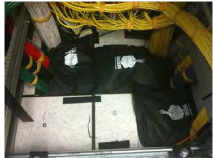
密封的电线穿墙 Sealed cable penetration
