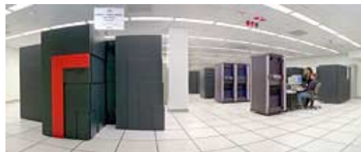
Figure 2 Supercomputers in LBNL's NERSC Center
