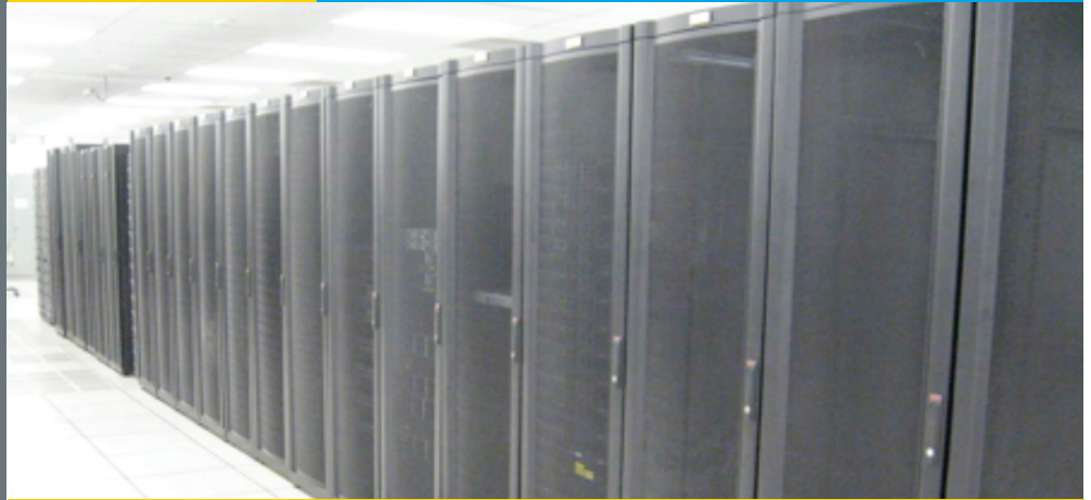
Figure 1: Extended Server Rack at SRS.
