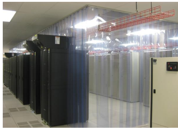
Figure 2. DC1 Hot Aisle Containment
