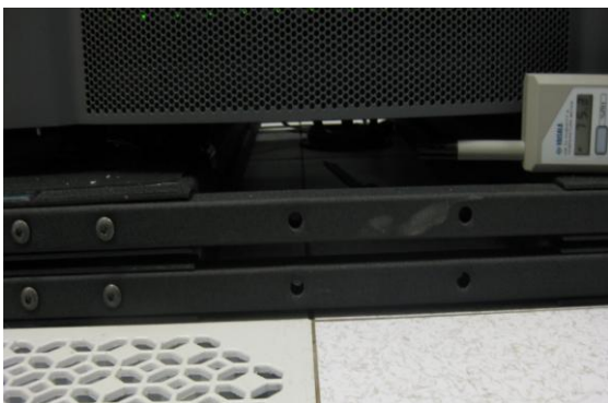
Figure 5. Air Recirculation Under the Racks
