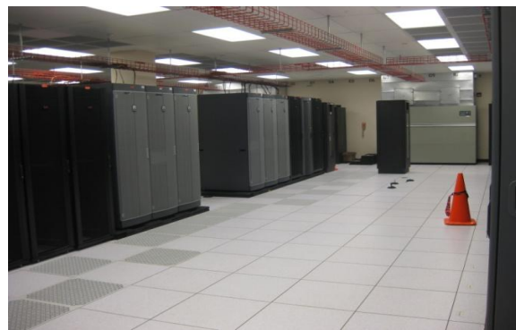
Figure 6. DC2 Lighting, and Perforated Tiles
