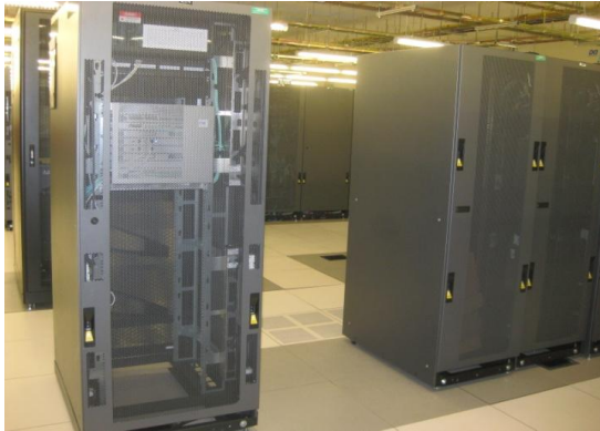
Figure 3. DC3 Openings in Racks
