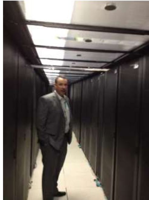
APC Hot Aisle Containment (with in-row cooling)
