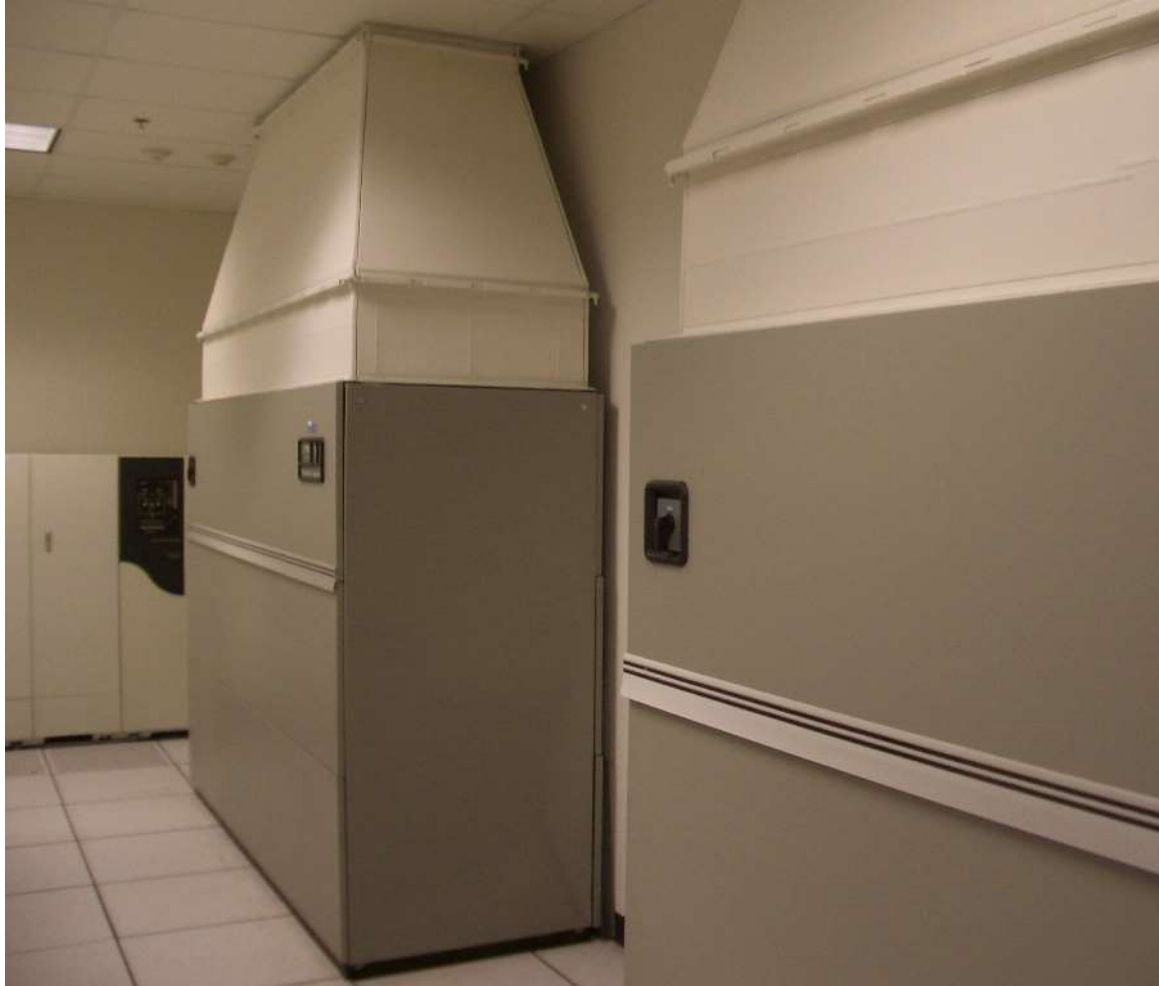
Return air duct on top of CRAC unit connects to the return air plenum.
