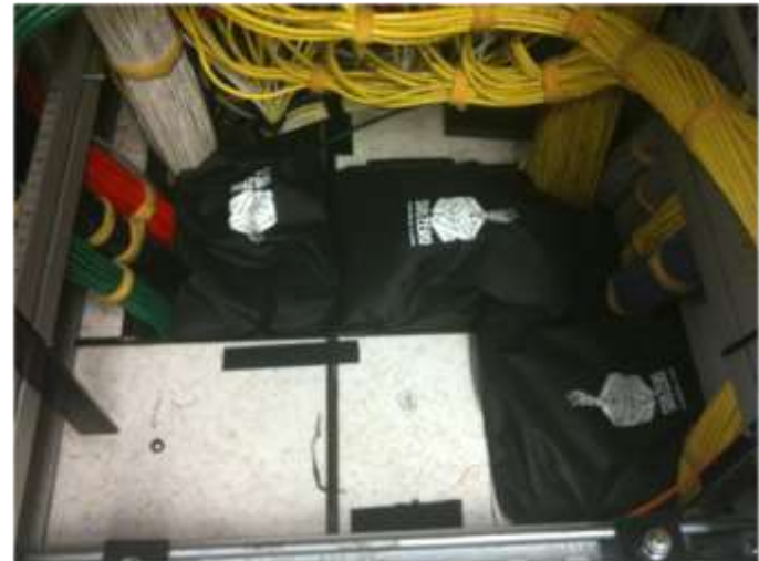
Sealed cable penetration
