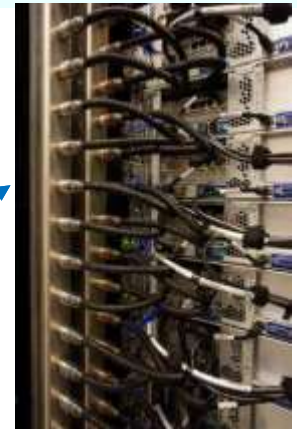
Traffic distribution unit manifold
