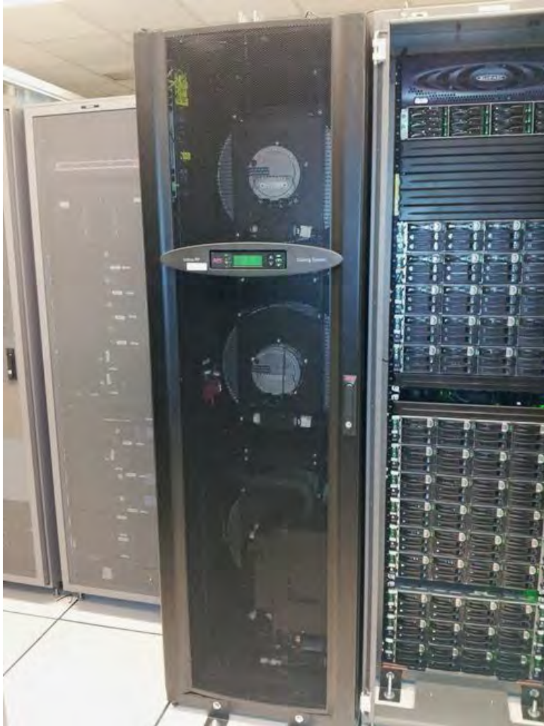
Figure 1-3: Prototype InRow™ Cooling Unit Installed at Lawrence Berkeley National Laboratory for the Demonstration
