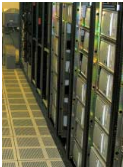
Figure 5. Data Center Racks
