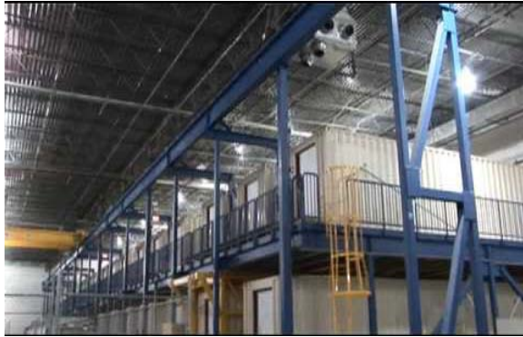
Figure 2: Data Center Featuring Container Units - Oregon
