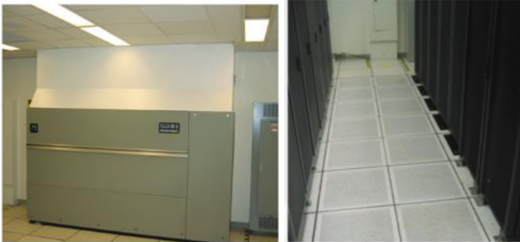
Figure 2. Improved air management. At left, CRAC unit with return duct from above-ceiling plenum. Today all but one of the seven original CRACs have been removed. At right, floor tiles with appropriate opening size to properly balance airflow.
