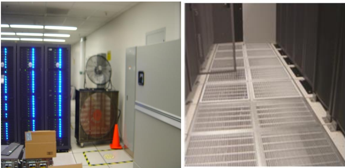
Figure 1. Air management issues in the early days. At left, portable fans were used to address hot spots; note CRAC with inlet from the space rather than above-ceiling plenum. At right, floor tiles with large openings addressed inadequate flow in this aisle but dropped the under-floor pressure, causing air deficiencies elsewhere.
