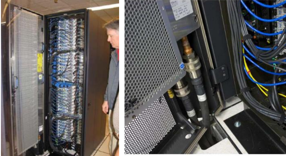
Figure 3. Passive rear-door heat exchanger (RDHX). At left, RDHX with door opened 90°. Hoses (at right) supply and return water from an under-floor distribution system.
