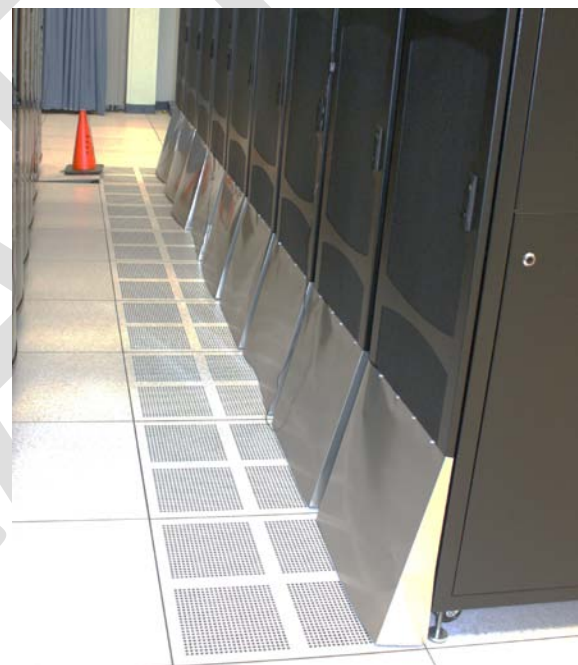
Figure 3- Hoods for Power Supply Unit air intake
