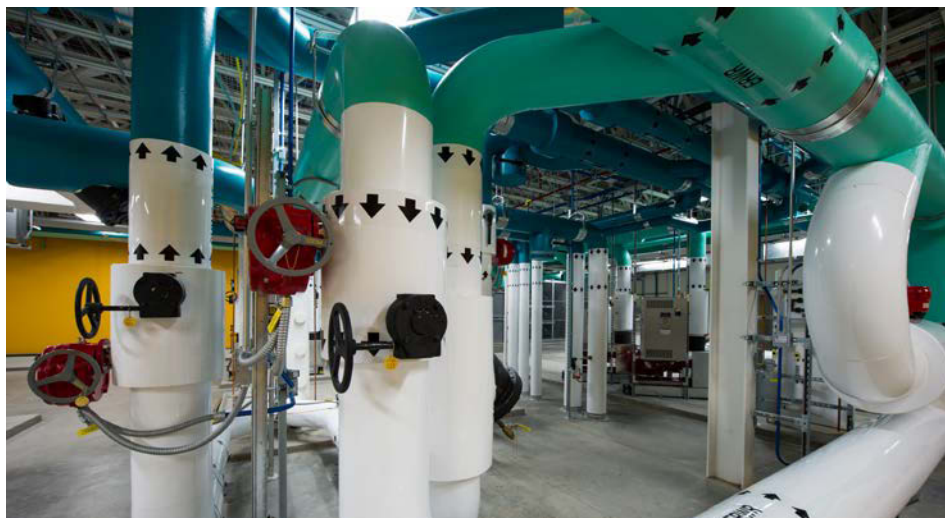
Photo by Dennis Schroeder, NREL 24645.
