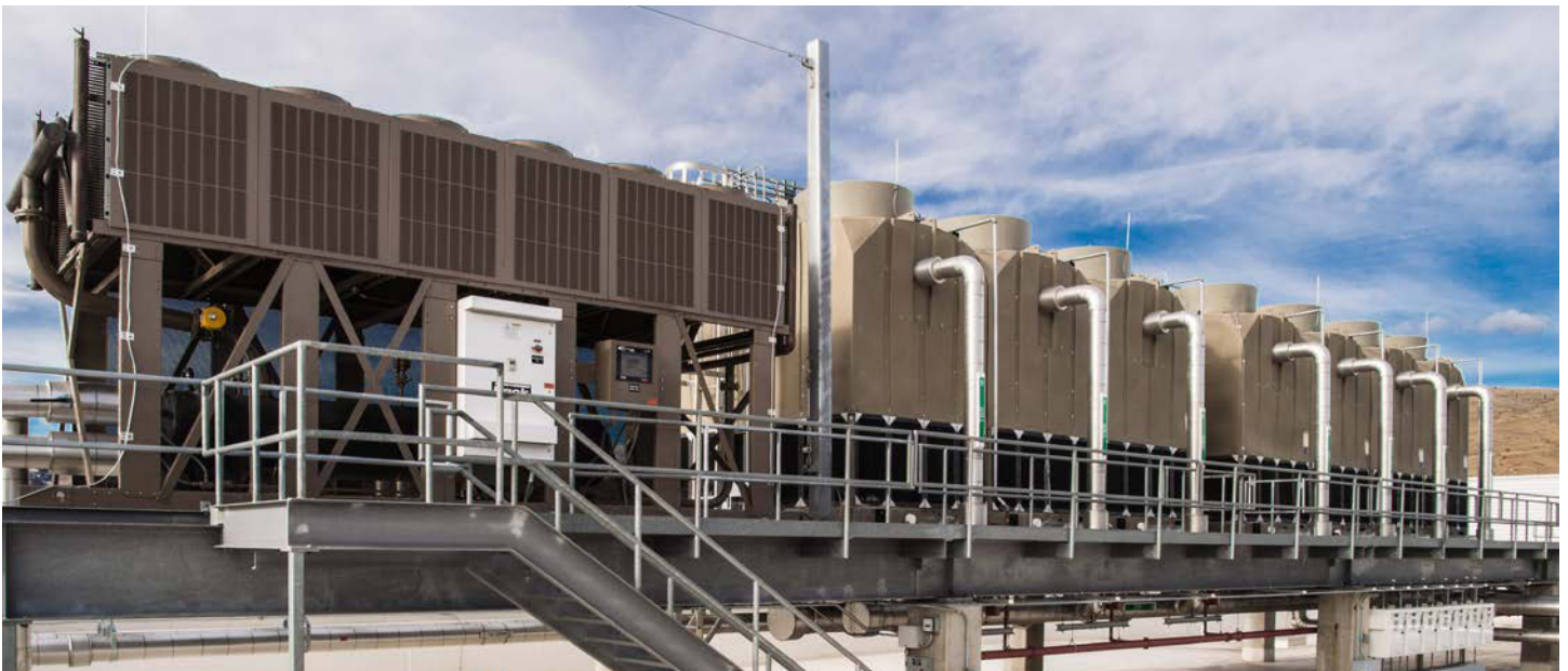
The thermosyphon cooling system sits on top of NREL's Energy Systems Integration Facility, which houses the HPC data center. The installation required only a 1-day outage to the data center. Photo by Dennis Schroeder, NREL 41999.
