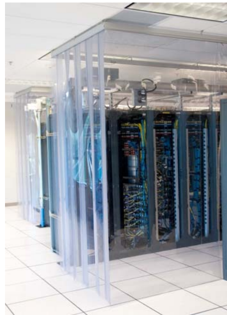
Figure 7: hot-aisle containment curtains.
