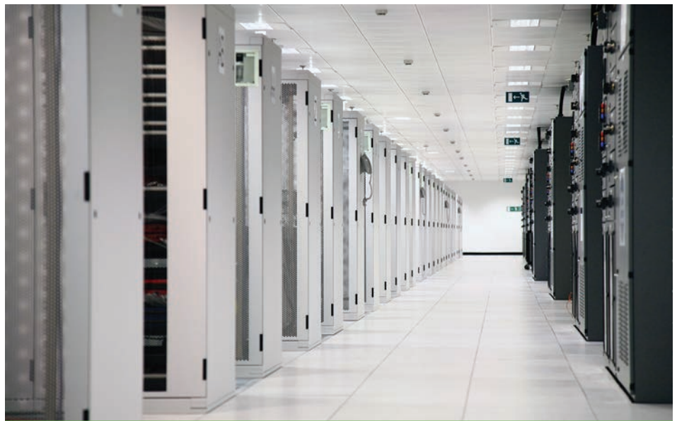
This server room in a data center displays server racks, power supply, and air handling systems. Photo credit iStock 1759899.
