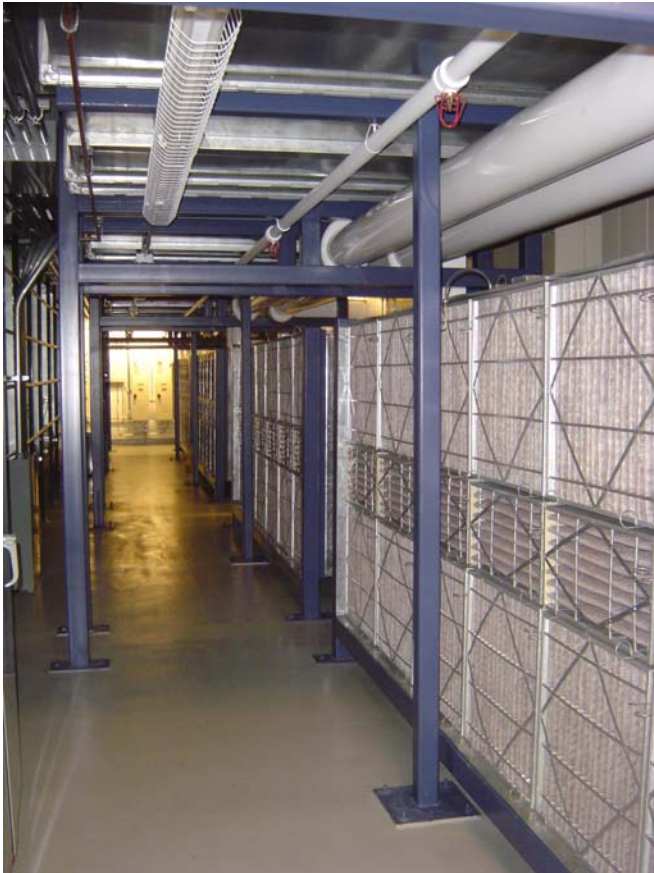
Figure 3 AHU return-air plenum
