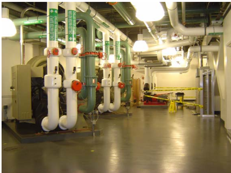
Figure 1 Chillers and chilled water pumps
