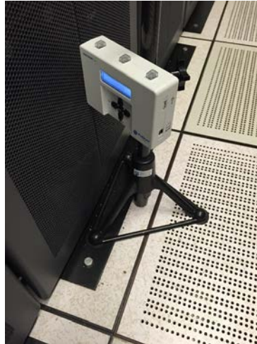
Figure 17. PurkayLabs: Seismic bracing. Units cannot be placed close to the rack fronts.
